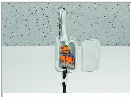
Pendant light connection in suspended ceilings
